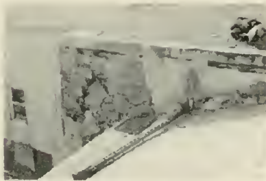
Figure 14. Corner of collapsing fire tower seen from adjacent roof
